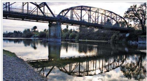
Historic or hazard? - Caltrans says the 88-year-old Healdsburg Avenue (Memorial) Bridge is overdue for replacement. Local citizens want to save it from demolition. - PHOTO BY ROLLIE ATKINSON
